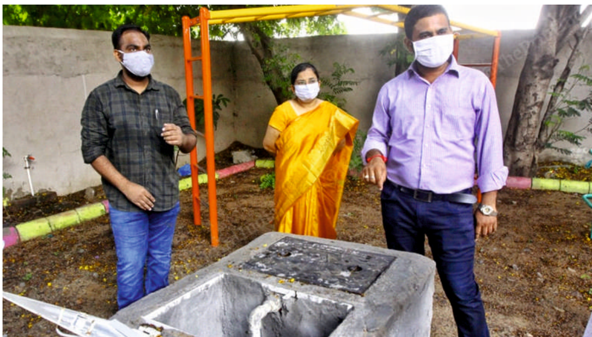
School authorities showing a rainwater harvesting structure in Vadodara | Praveen Jain | The Print
